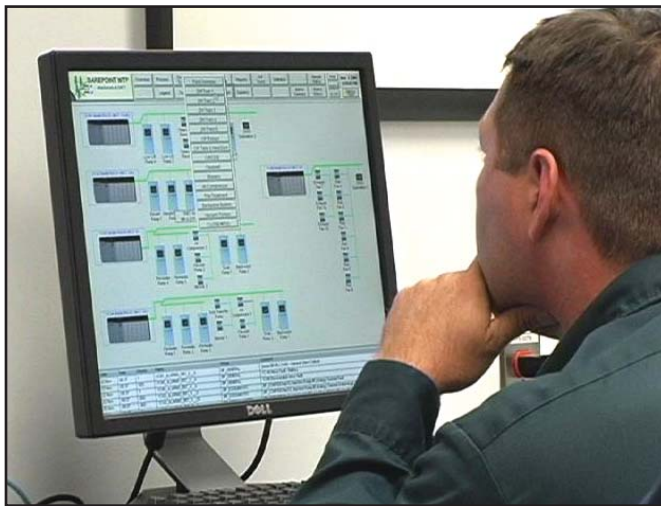
Operators can stay in the control room and monitor all plant processes and analytical equipment from there.
