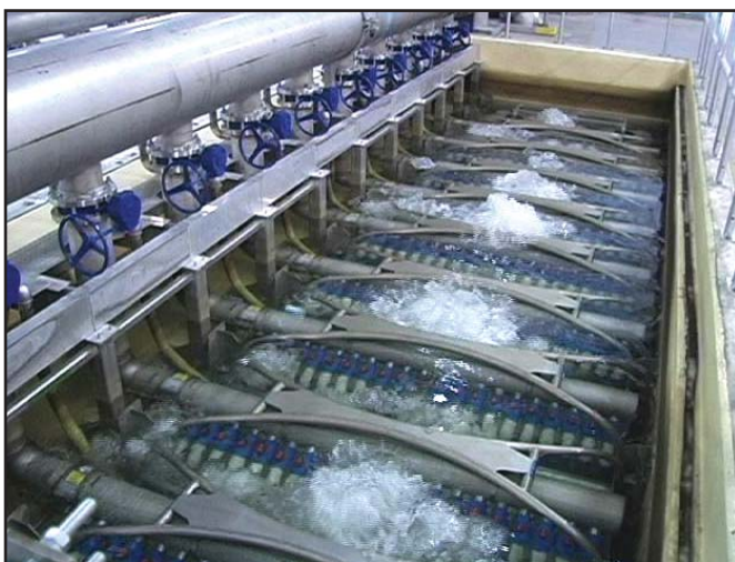
Backwash cycle on the Ultra Filtration trains.
