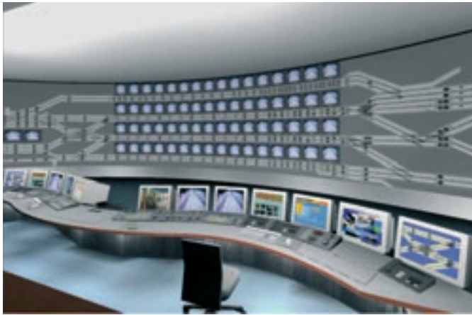
Central control unit
