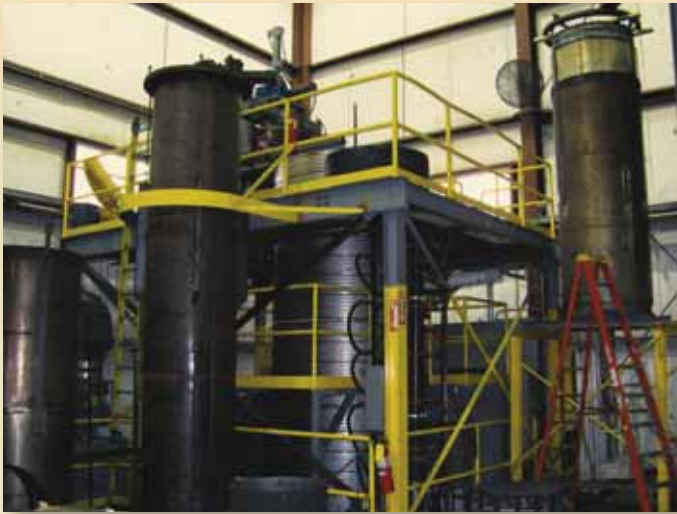
Figure 3: Bodycote plant floor showing control of kiln.
