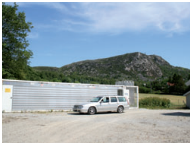
In this plant at Aksdal, a short distance outside Haugesund, is a tank which contains LNG. The liquid passes through evaporators, where it is converted into gas before being delivered to users.
