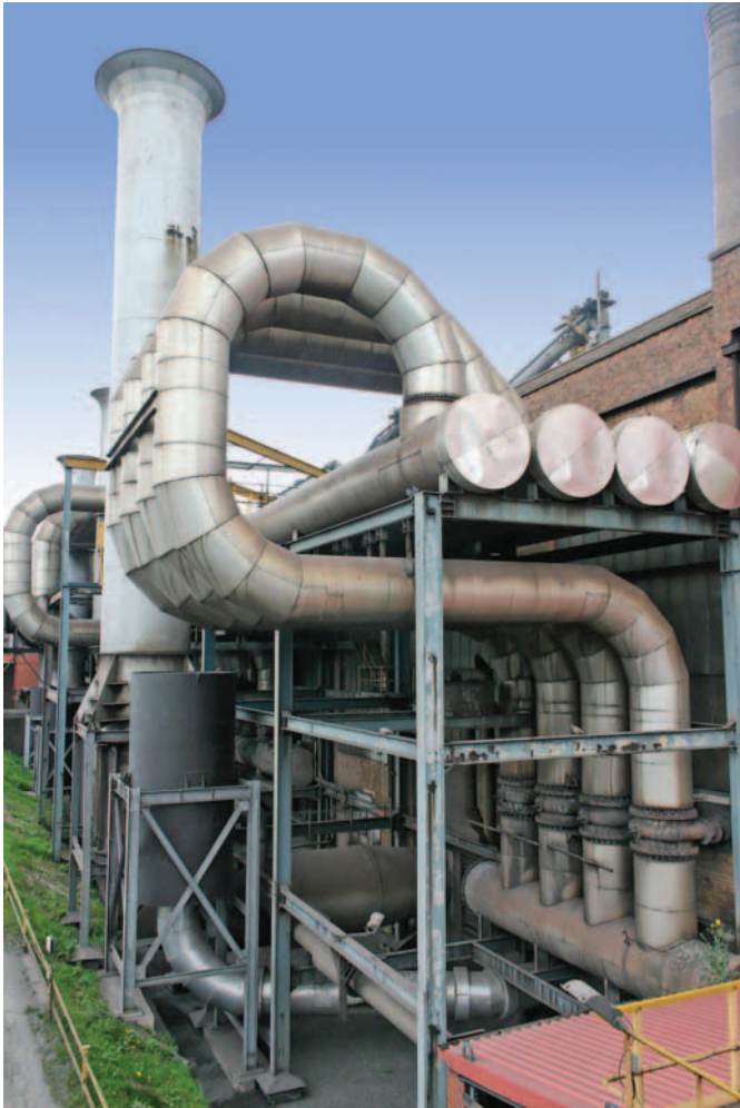
Air intake and blast manifold
