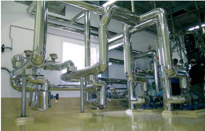
PURAC plant in Montmeló
